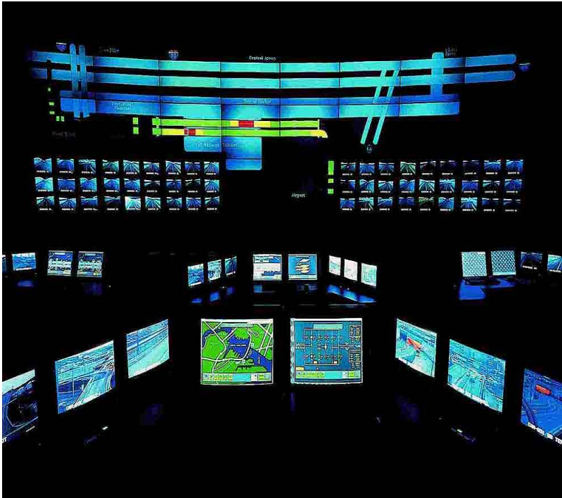
The Central Artery/Tunnel Project's Operations Control Center (OCC) in South Boston contains the most advanced electronic traffic monitoring and incident response system in the world. (photo credit: Massachusetts Turnpike Authority, with permission)
